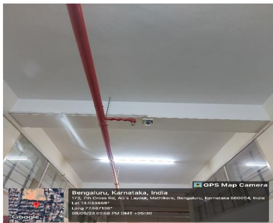
CCTV IN CORRIDOR
