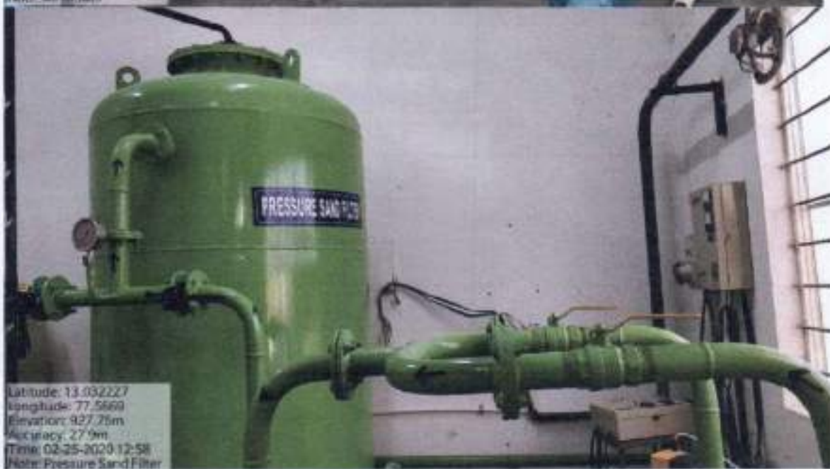
Time: 02-25-2020 12:59 Note: Air Blower
