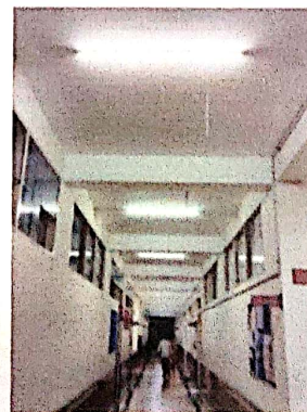
LED bulbs and tubes in the corridor
