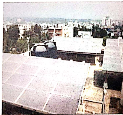
Solar panels installed on the building
